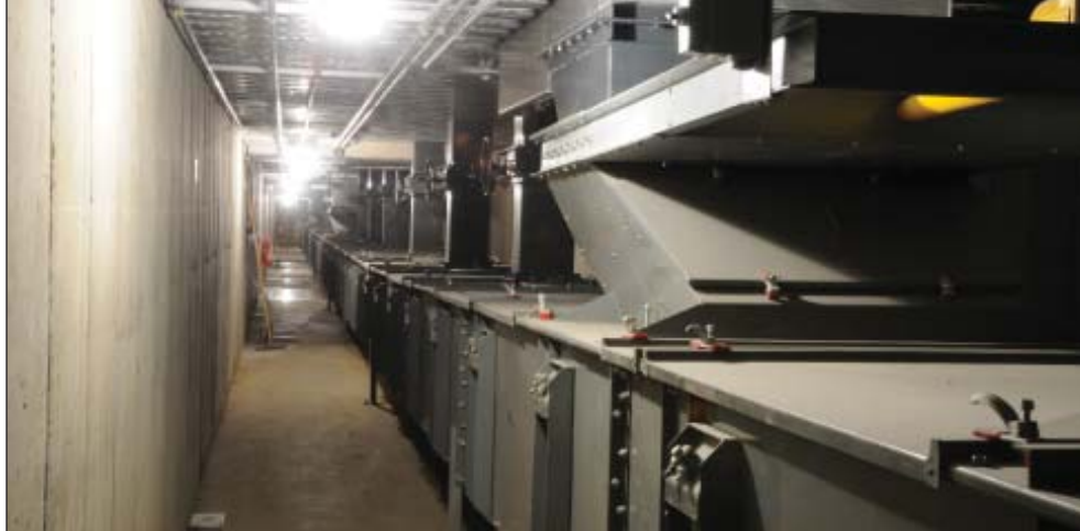
Series of 60,000-bph Hi Roller enclosed belt conveyors in a below-ground tunnel reclaim grain from 375,000-bushel SCAFCO tanks.
