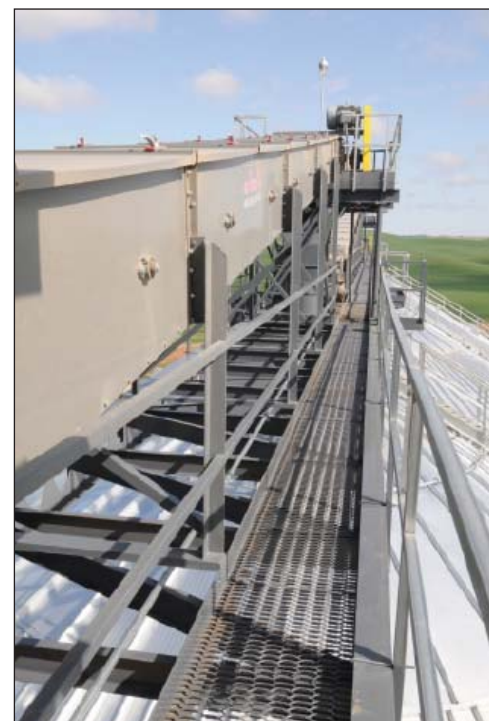
Overhead 40,000-bph Hi Roller enclosed belt conveyors carry grain out to storage.
